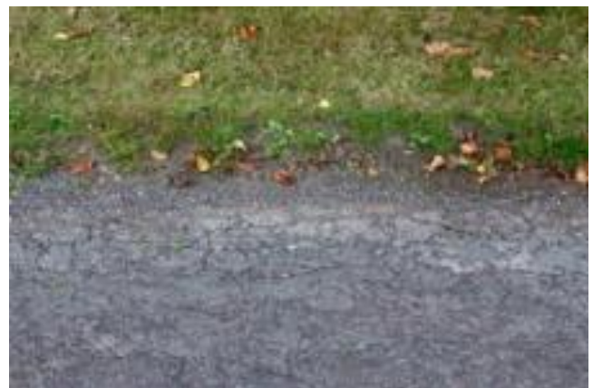
Start of cracking due to no hard edge at grass verge.
