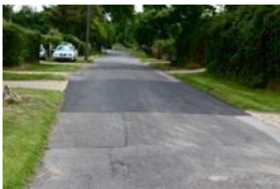
When monies available a large strip is repaired with new foundation every couple of years
