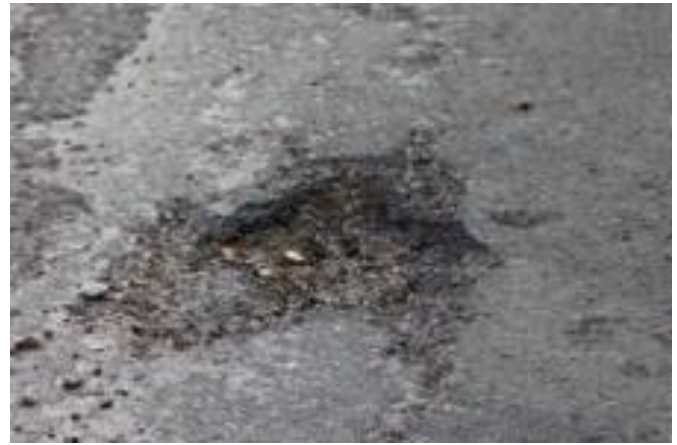
Small pothole being monitored by the committee
